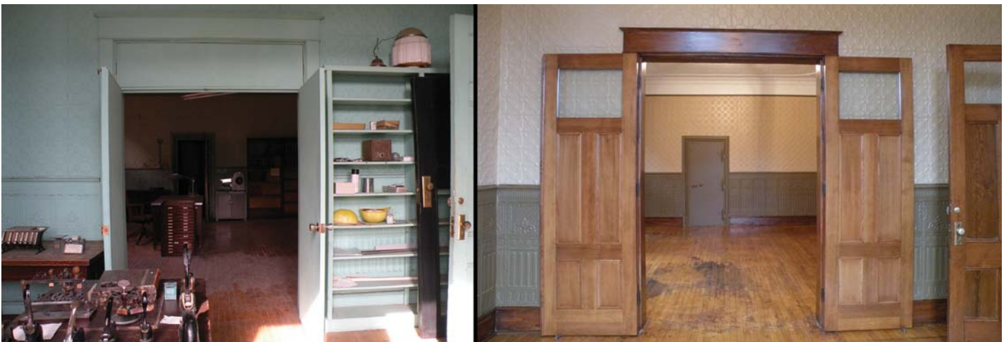
The historic clerk of court's office before and after restoration in fall 2015. The two doors in the center were custom made to match the existing historic doors throughout the building. This office will be named the Mary Faith Young Room in memory of the 1883 Stutsman County Courthouse Committee founding member who passed away in November 2015.
